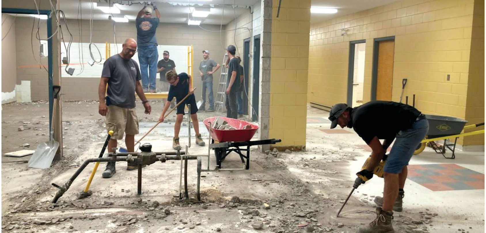
Volunteers capably help in Smithville with the demolition and prepare for the renovation.
